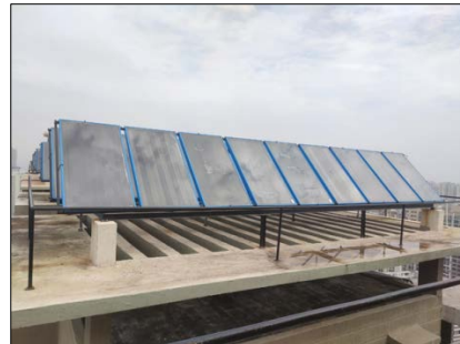
Solar Hot water Panels
